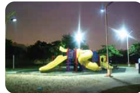
Solar Park Lighting AMERICAN UNIVERSITY, Sharjah, UAE
